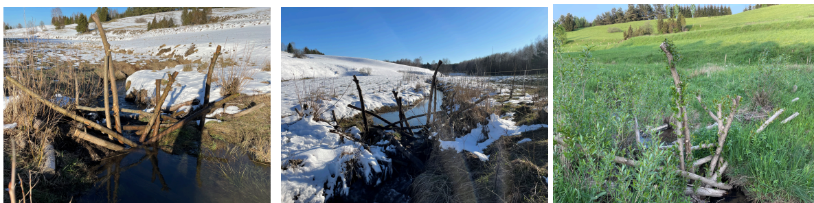
Beaver Dam Analog blocking drainage ditch in Bieszczady, using willow shoots - from building in autumn to the next summer. Photo credit Andrzej Czech
