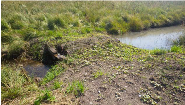
Example of damming culvert (photo credit D. Horabik)
